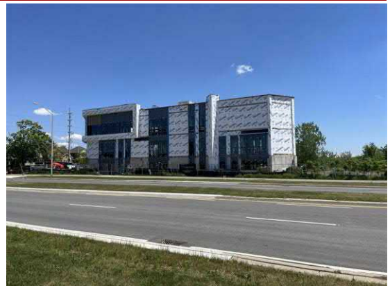
Picture 14: View of a building undergoing construction south of the Site, facing southeast.
